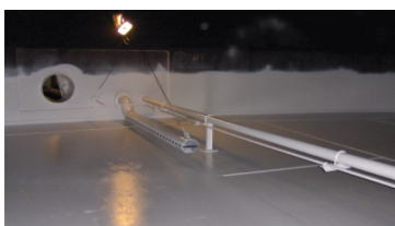
Interior crude oil storage tank
